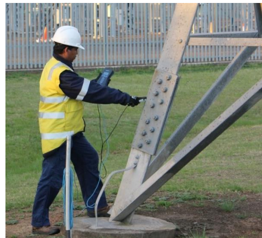
Measuring touch voltages during an injection test with the Safearth MI1 Tuneable Voltmeter
